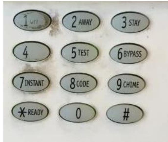
Dirt and wear on a keypad
